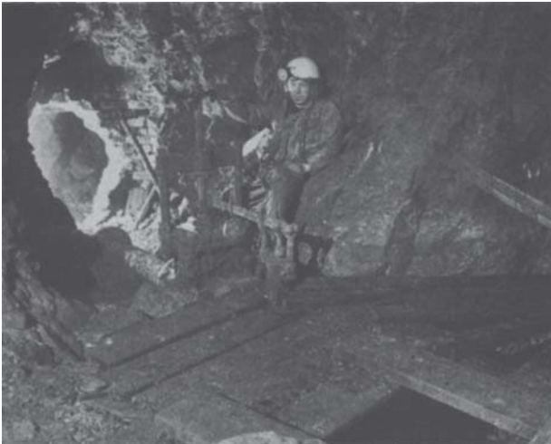
PLATE IV. GREENSIDE MINE. THE STOP AND BLOW-OFF VALVES AT HEAD OF CLIMBING WAY, HIGH HORSE LEVEL. ONE OF THE BREACHED DAMS IS VISIBLE TO THE LEFT. (PHOTO: R.H.B.)
