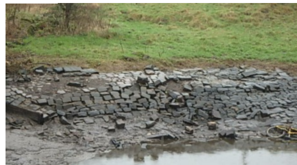
Photo 2:-The sets at the side were not considered to be in too poor a condition to rebuild them Along the route are mile markers originally used to calculate tolls for cargo being carried along the
