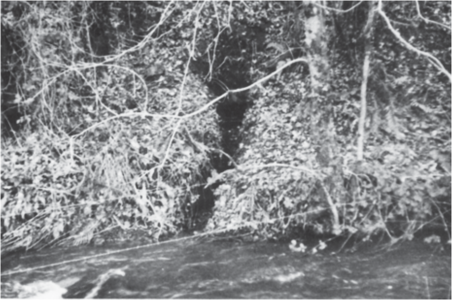
Plate I. South Exmouth & Hennock. Portal of the drainage adit, about 50 yards downstream of Hyner Bridge. Now partially choked, it nevertheless still emits a steady flow of water from the flooded workings of Hennock and South Exmouth mines.
