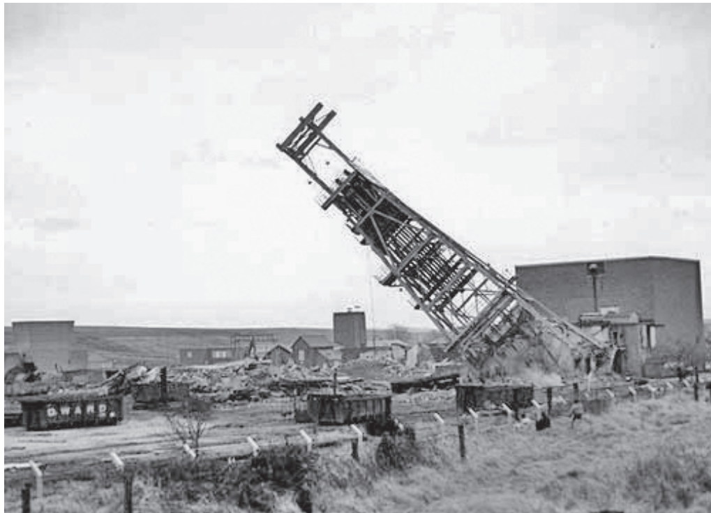
Figure 68. Demolition of Newstead Colliery, Nottinghamshire [Photograph courtesy of Shane Phillips © Creative Commons licence 2.0].
