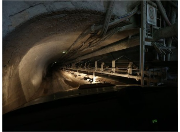
Materials handling conveyor.
