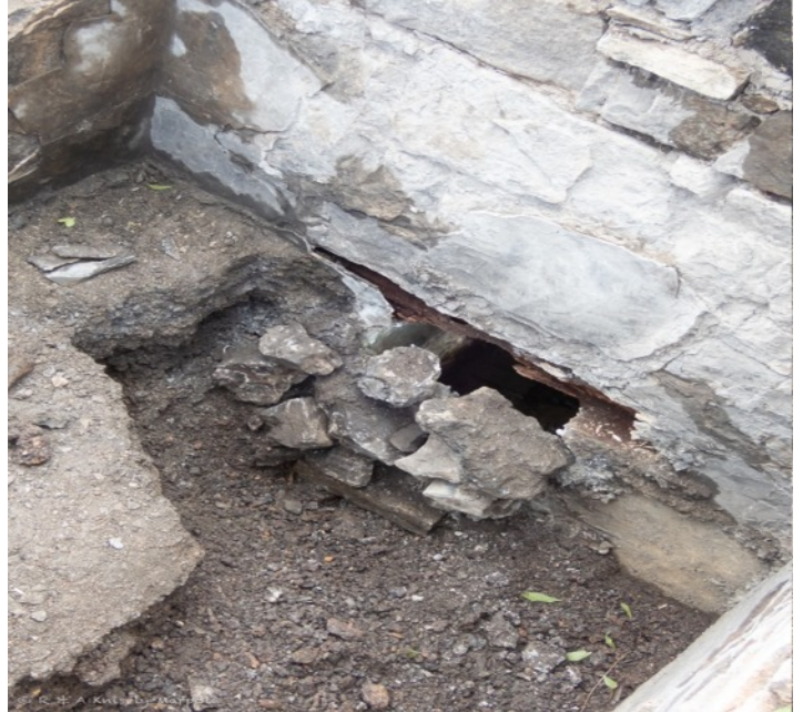
In bin two, this drystone wall closed off the arched exit tunnel.
