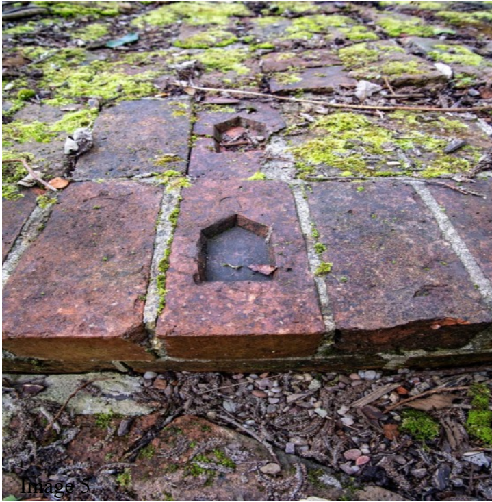
The two arrows in the brickwork. I am taking this to be the position of the flue in the North section of the chimney
