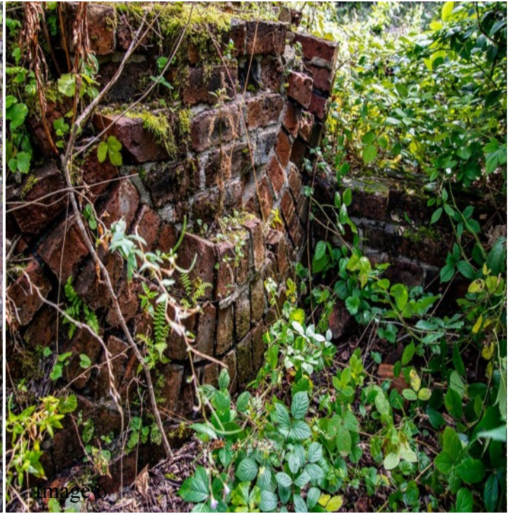
The arch for the flue in the South West section of the chimney. The bricks inside the arch were added during the 2014 archeological dig {for support}. The wall running at 90 degrees to this arch is a kind of buttress which joins an external wall that supports the chimney.
