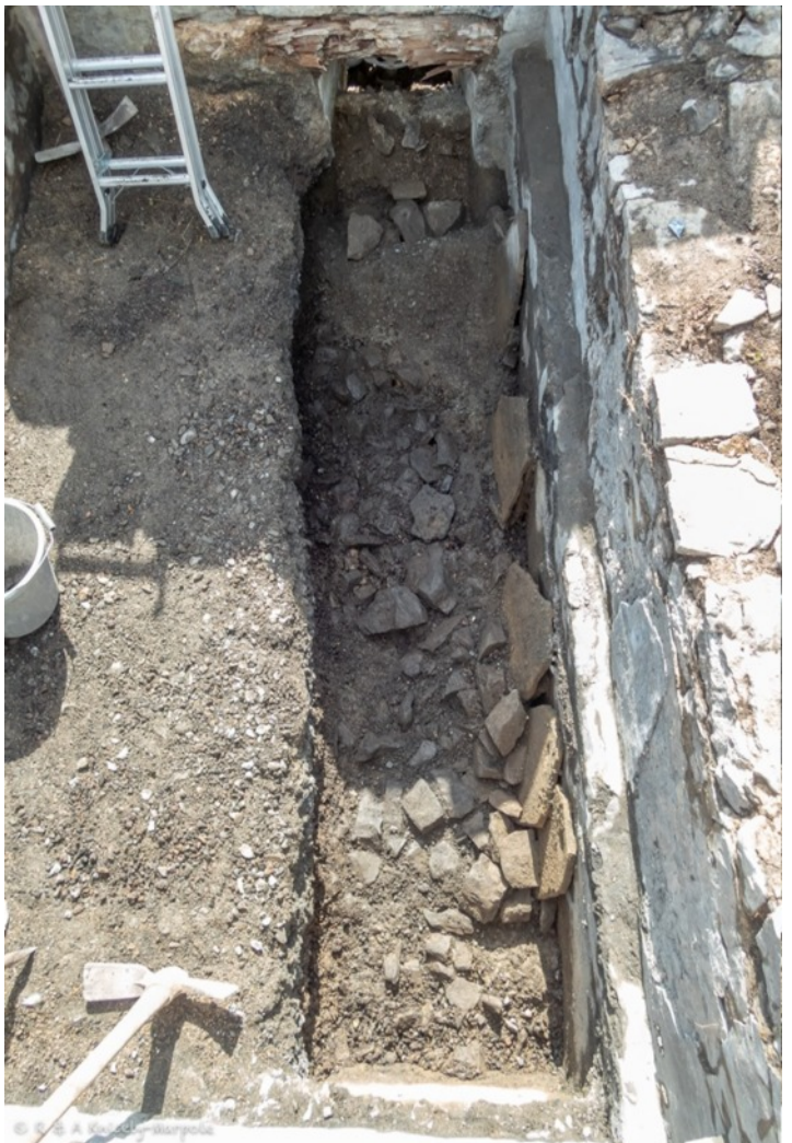
A level was reached where it was thought it was best to take out a half section to determine how far we needed to go down. The roofing stones laying against the wall were extremely puzzling! Left Roofing stones found in the bin.
