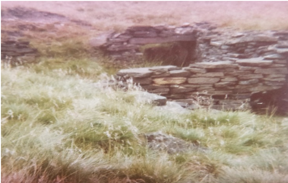
Intake Colliery 1979. The main drift is at the top. The hole in the wall was to let the water out.
