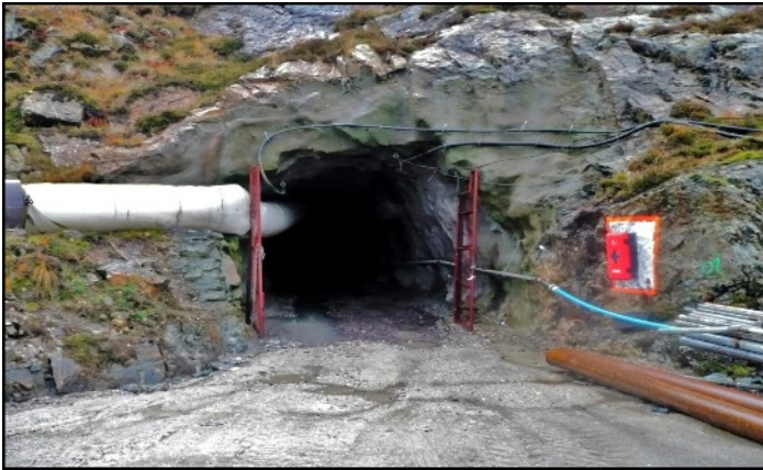
The entrance to the adit, which is now strongly reinforced for safety reasons in an illustration provided by Scotgold Resources.
